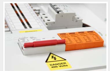
SPD mounted beside main switch
